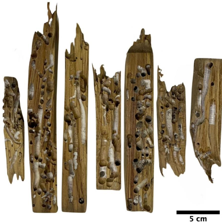
Fig. 9. Damage to wood caused by marine borers at Jikomalamo Beach, Takome Village, West Ternate Sub-district.
