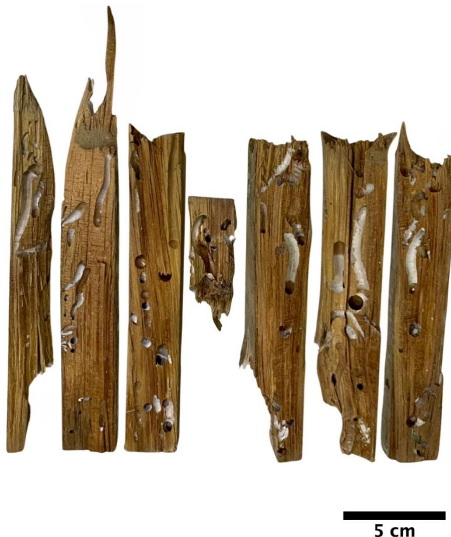
Fig. 8. Damage to wood caused by marine borers at Ake Rica Beach, Rua Village, Ternate Island Sub-district.
