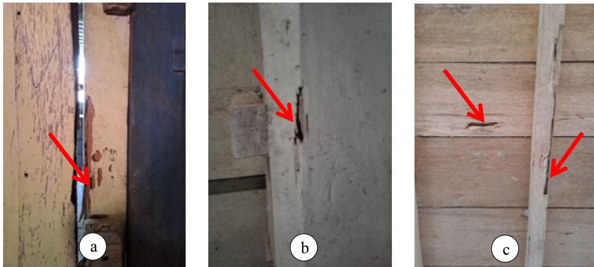
Fig. 3. Damage and open galleries caused by drywood termite attacks on (a) door frames, (b) pillar connecting beams, and (c) floors and floor supporting beams.
