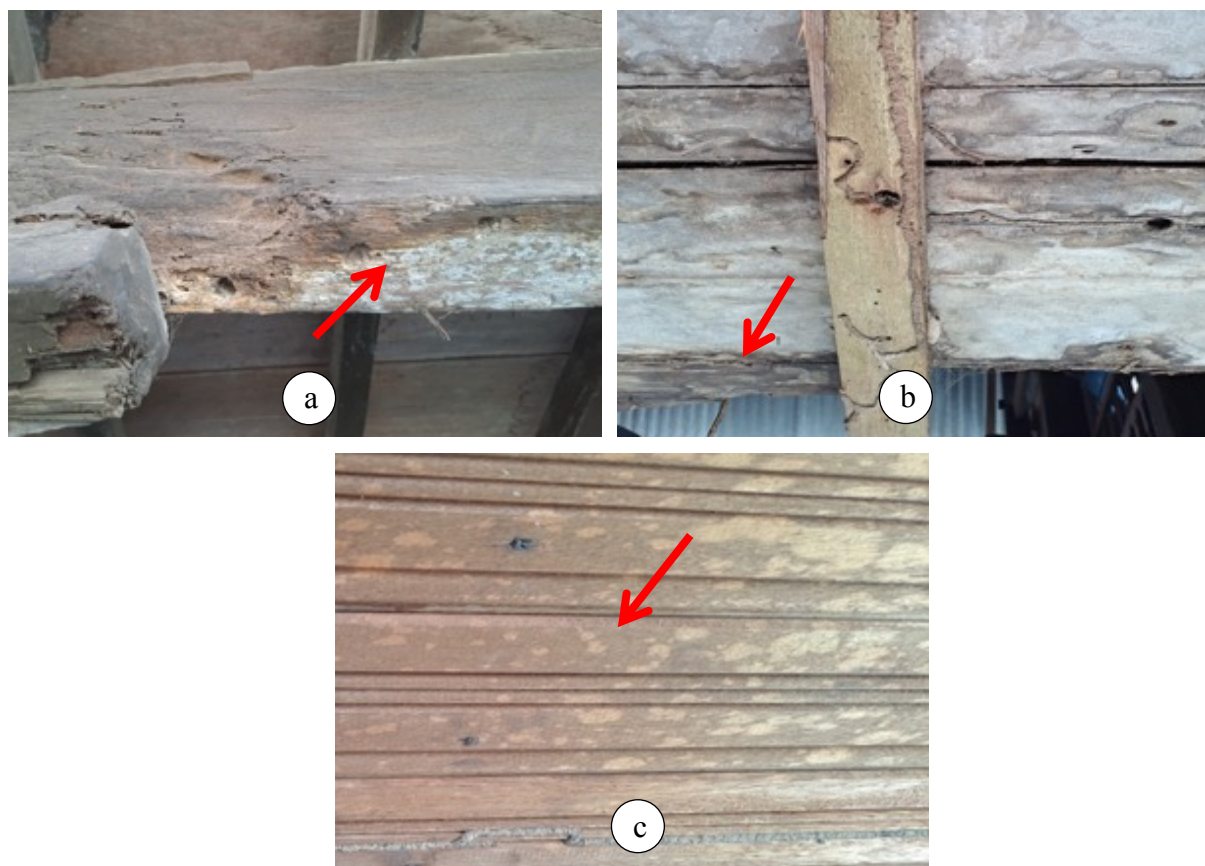
Fig. 8. Biodeterioration symptoms are caused by wood-decaying fungus on (a) the beam connecting the pillars, (b) the bottom surface of the floor, and (c) the ceiling.
